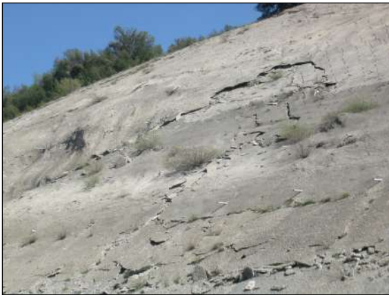
Figure 6. Superficial cracked shotcrete
