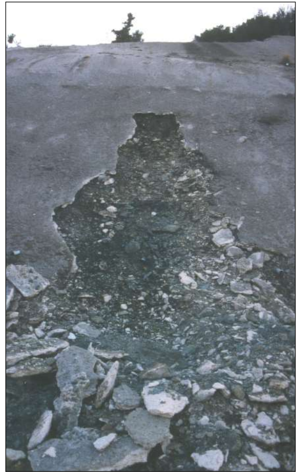
Figure 7. Thin shotcrete cover of Flysch material
